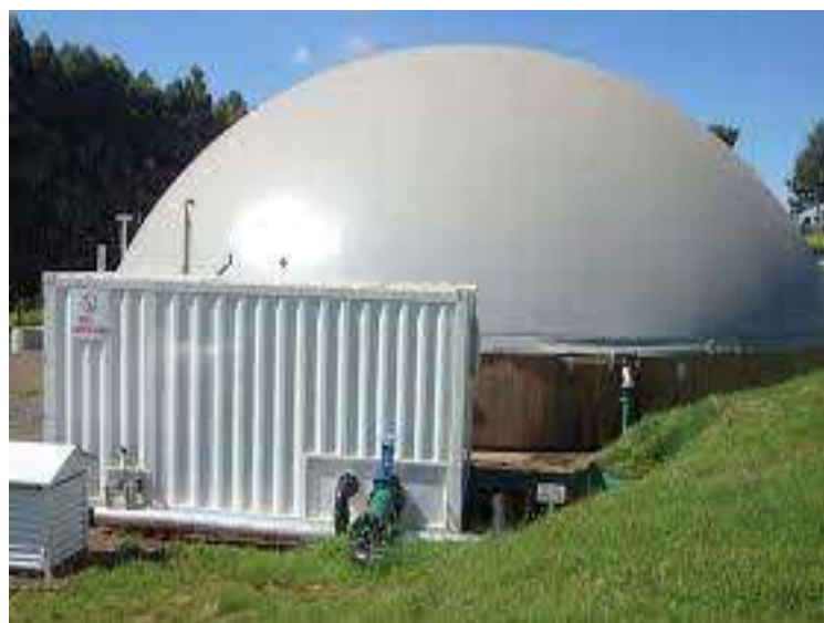
Figure 6: Biogas production unit Source: Finlays.net
